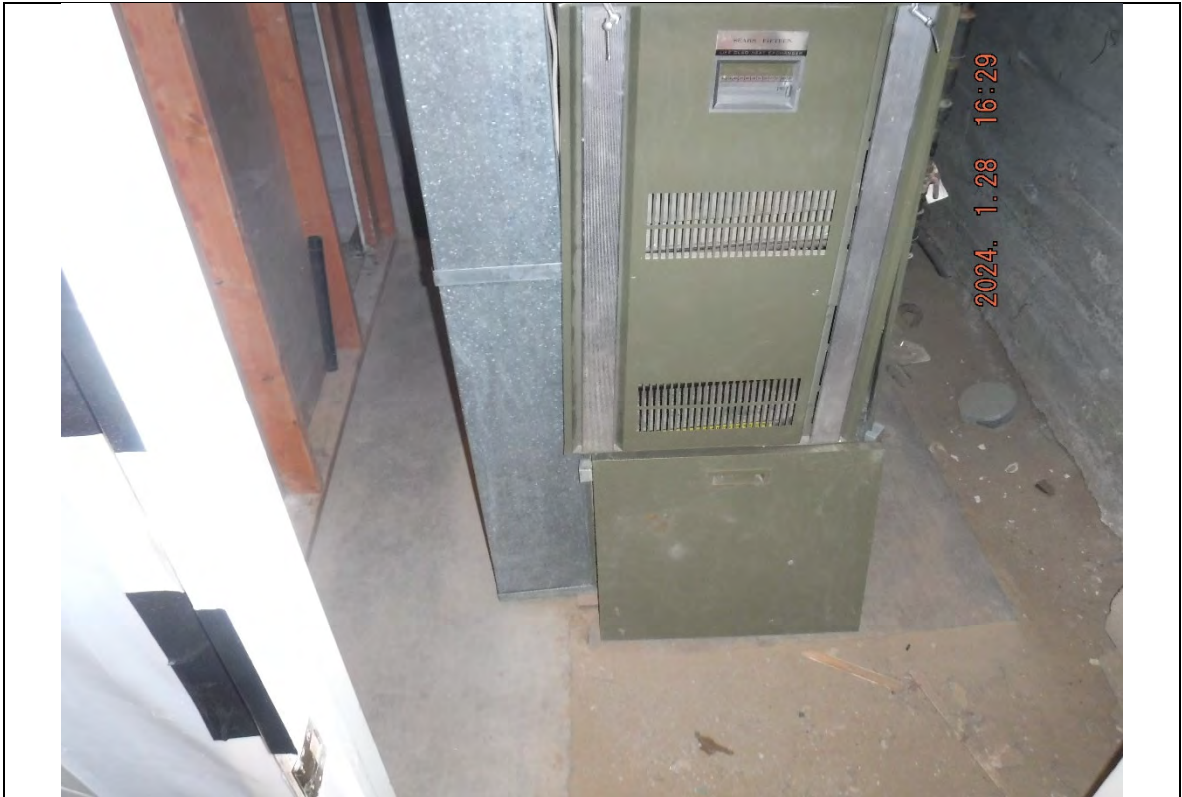
Photograph: 2270 Furnace room, following final cleaning, facing south (exposed earthen areas shown at bottom right).
