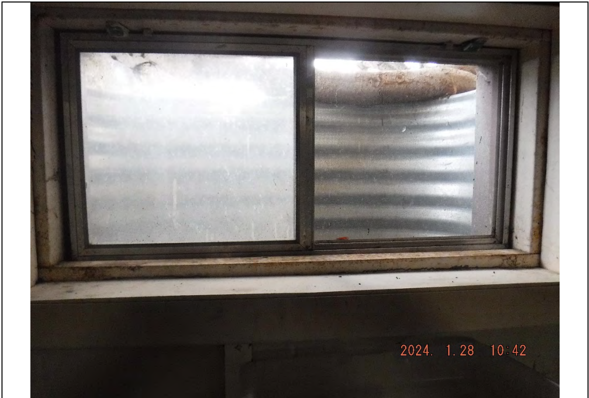
Photograph: 2257 Basement window sill, following initial cleaning.
