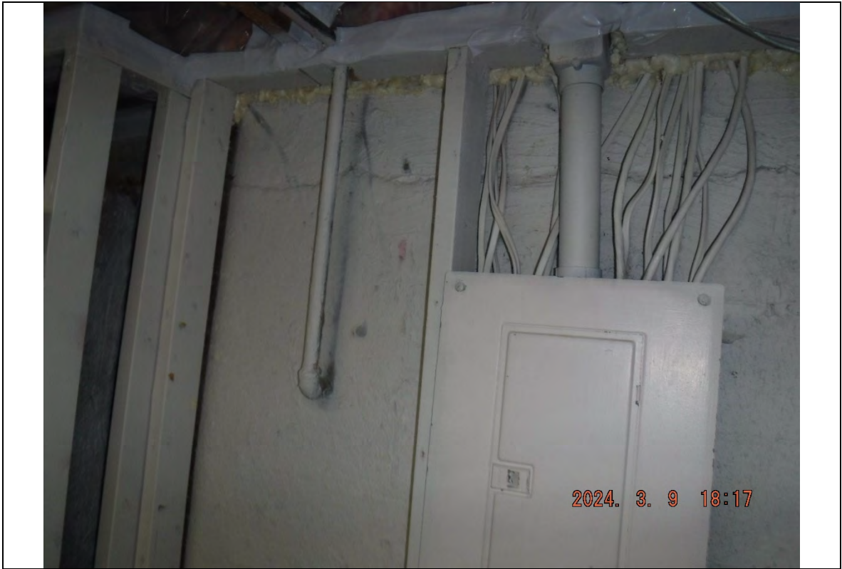
Photograph: 2446 Smaller pathways were sealed with insulation foam, north side of basement, facing north.
