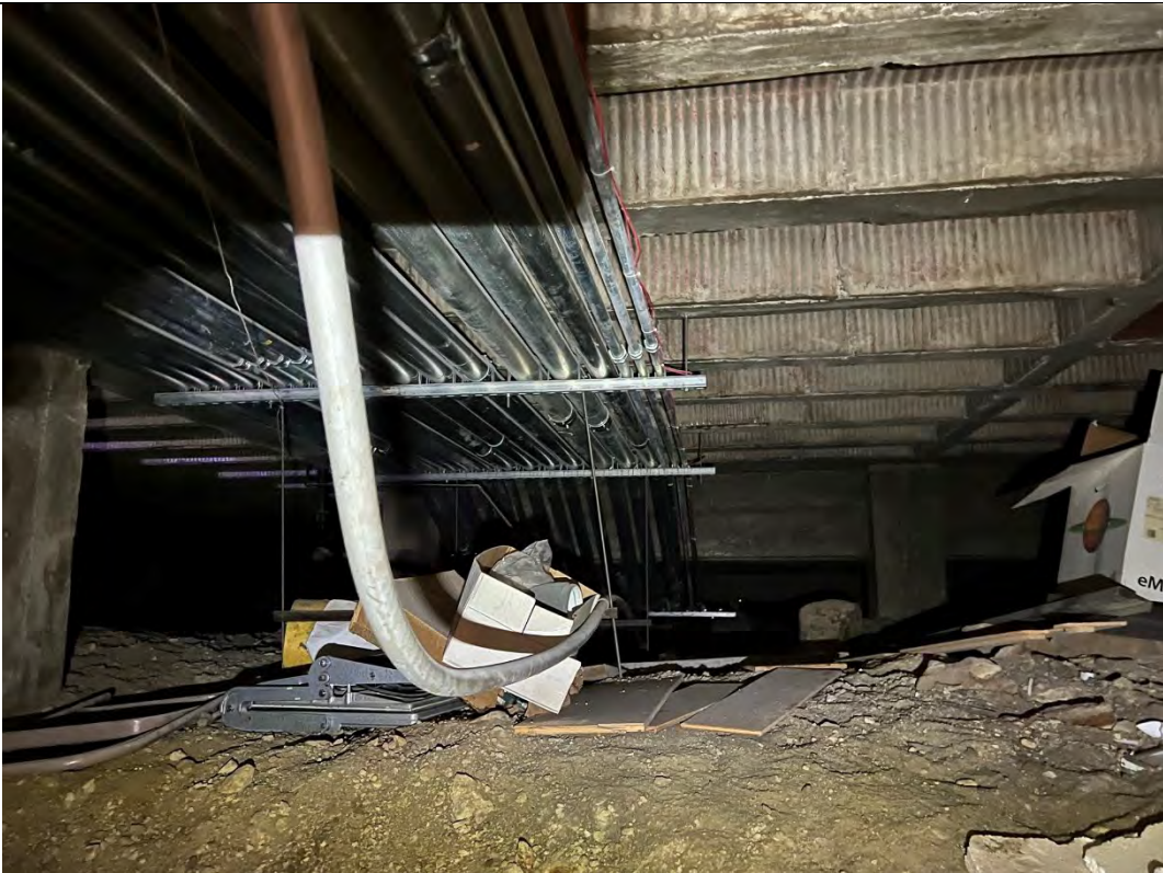
Photograph: 5 Refuse in south east crawl space entrance. Approximately 2-3 cubic yards of material was removed.
