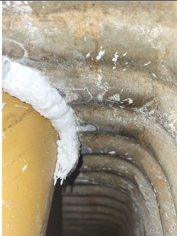
Photograph: 7 Openings around pipes in crawl space were sealed with insulation foam.
