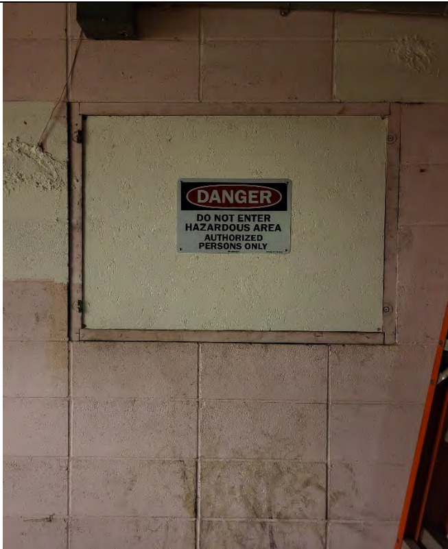
Photograph: 11 South crawl space entrance, sealed with screws and attached aluminum sign stating "Danger: Do Not Enter Hazardous Area Authorized Personnel Only".
