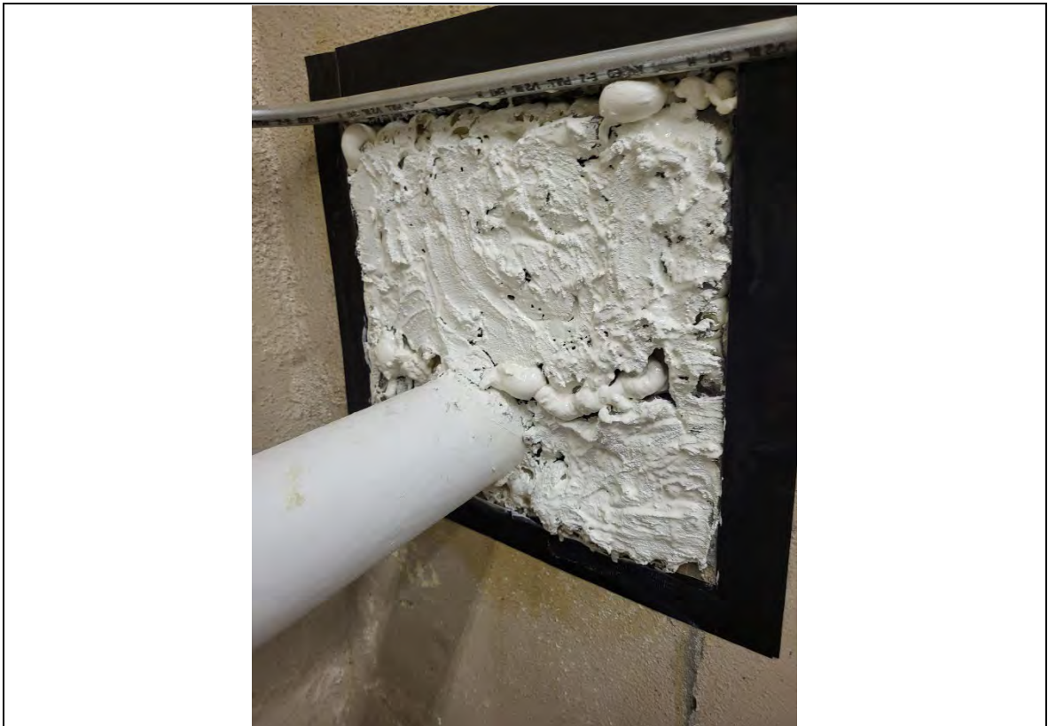
Photograph: 16 Large hole in boiler room, sealed with combination of wood, DAP, and insulation foam.
