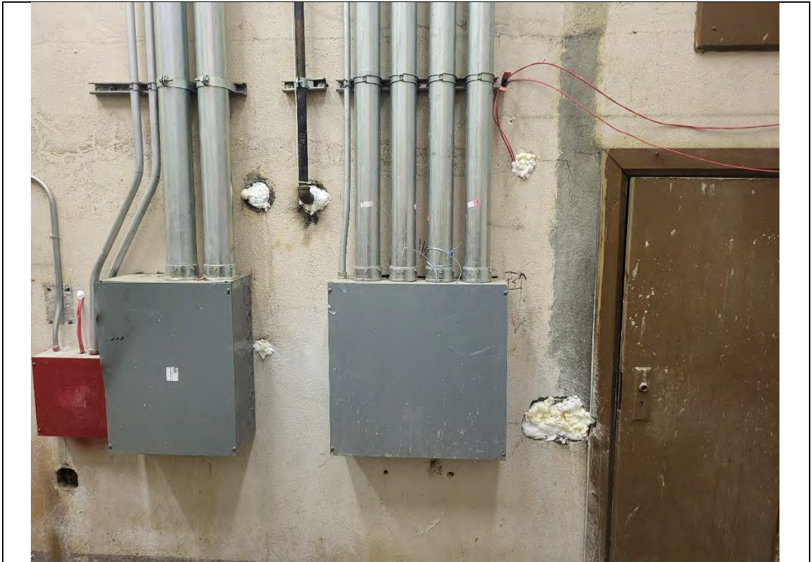
Photograph: 9 Smaller holes were filled with combination of insulation foam and DAP concrete patch.
