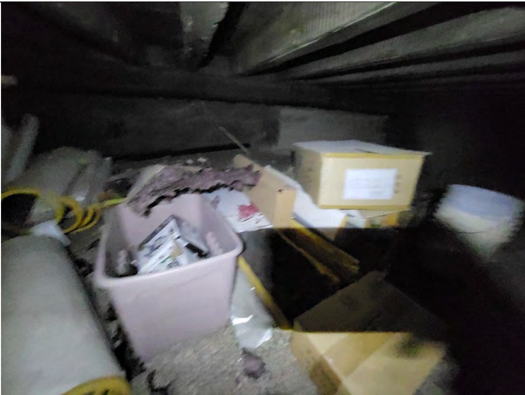
Photograph: 2 More refuse located deeper at north entrance of crawl space.
