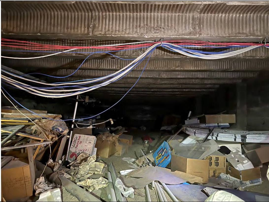
Photograph: 3 Refuse in southwest crawl space area. The southwest crawl space was completely full of refuse and it took the field team all day Tuesday and Wednesday morning to remove all materials. Approximately 40 cubic yards (filled 4 10 yard dumpsters) of material was removed from this area.
