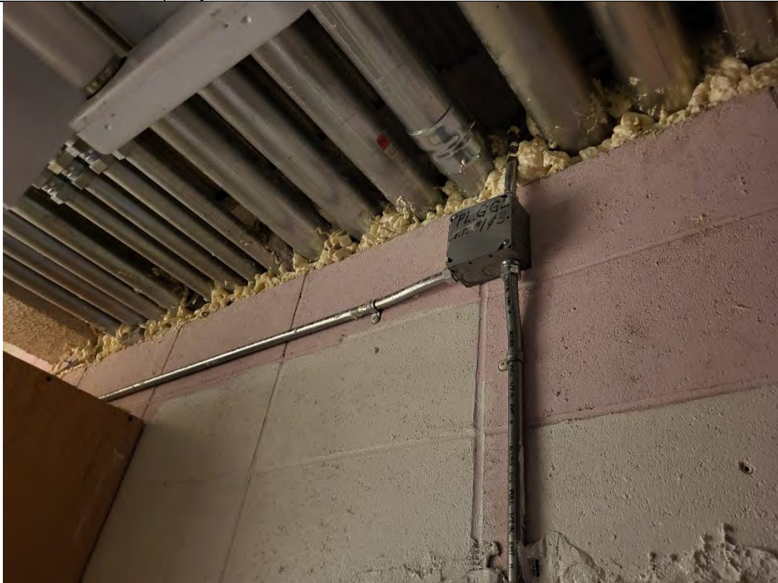
Photograph: 12 Large gap above southern crawl space entrance, sealed with DAP and insulation foam.
