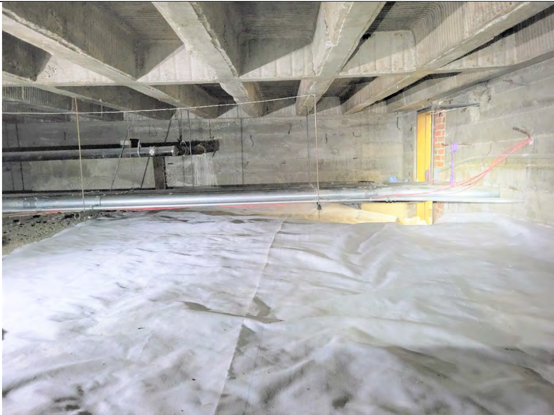
Photograph: 21 View from east corner of crawl space entrance by boiler room, with geotextile fabric, facing west. Door entrance is on the right in the photograph.
