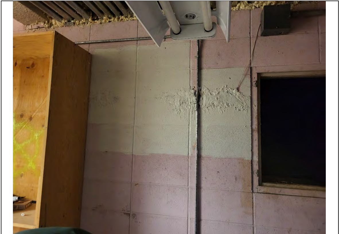
Photograph: 15 Two large holes, next to southern crawl space entrance, sealed with DAP.
