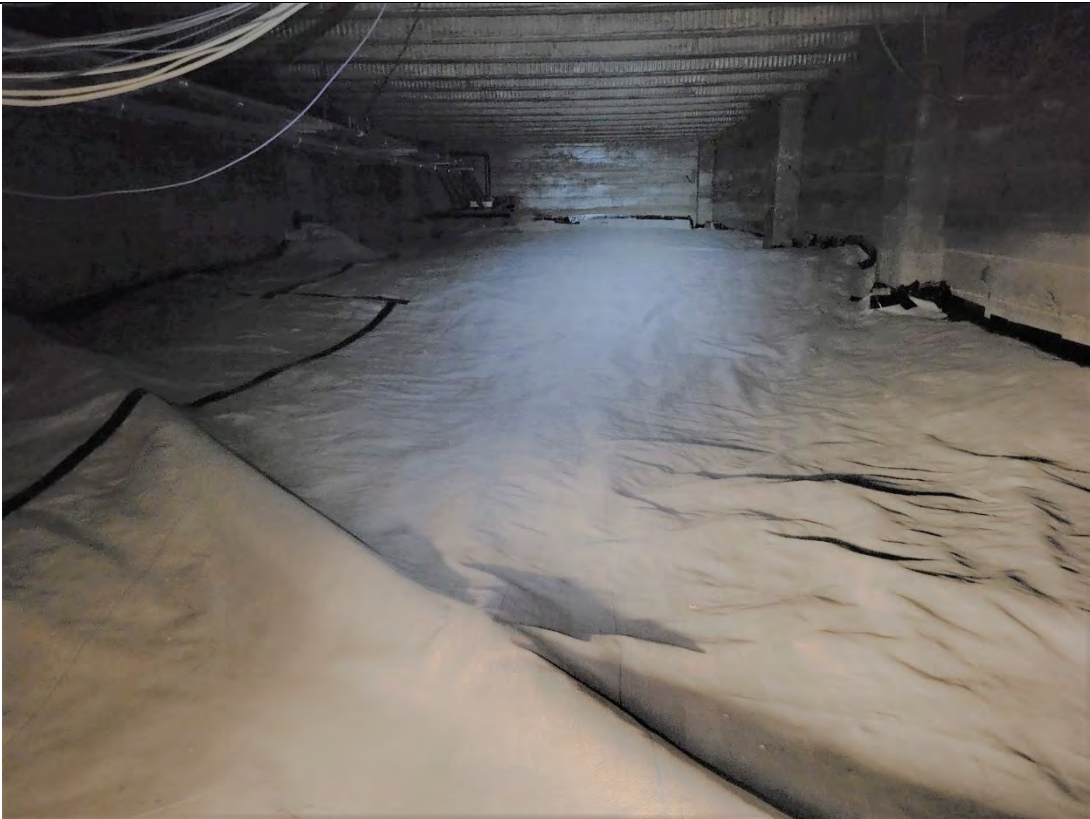
Photograph: 19 View from southwest crawl space entrance, with geo-textile fabric fixed to ground, facing west. Existing pipes created "bumps" on fabric surface.
