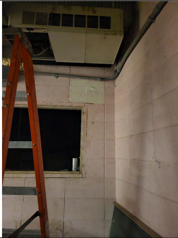
Photograph: 13 Hole above southern crawl space entrance, sealed with DAP and painted.
