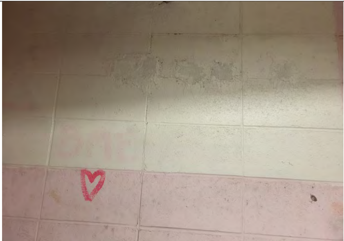
Photograph: 14 Four holes next to southwest crawl space entrance, sealed with DAP and painted.
