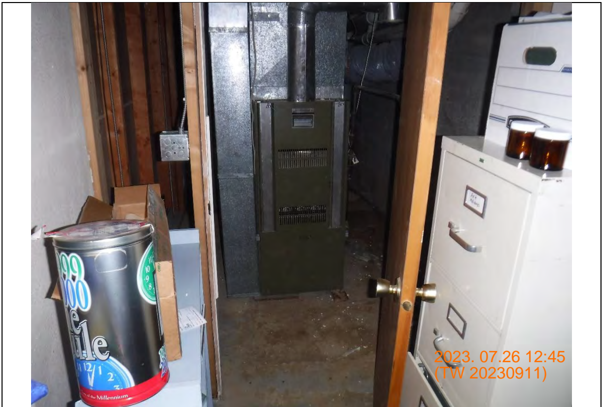
Photograph: 1726 View of furnace room entrance, facing south. Exposed earthen area is at the base of the boiler. 7/26/2023 12:45
