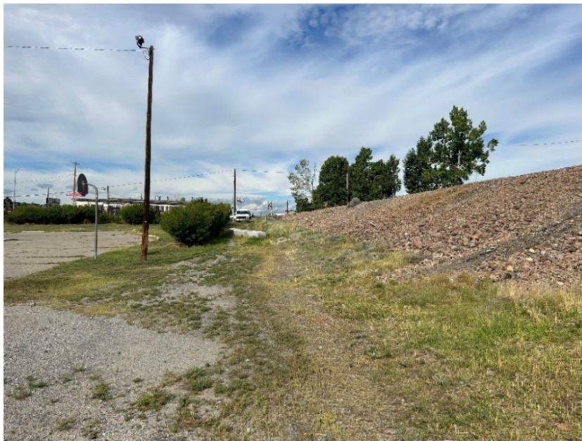
Photograph 1: South slope of railbed, facing west toward Montana Street, exhibits rilling and staining.
