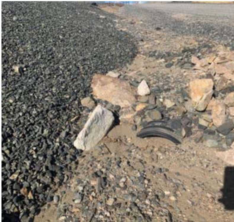
LY-HDPE-02: Sediment accumulated at pipe outlet. Sediment removal is part of the 2021 inspection maintenance items scheduled.
