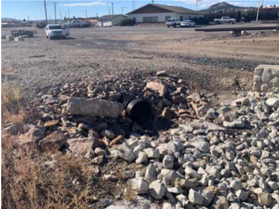
LY-D-01: Sediment accumulation.
