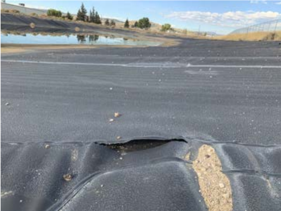
LY-PND-01: New tear in liner (Two liner tears from 2021 inspection still present).
