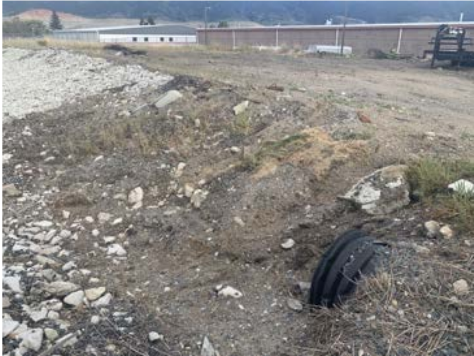
MY-D-03: On the south side of the northeast ditch at MY-HDPE-03 outlet, 1-3 inches of sediment is covering rock over an approximately 60 SF area.
