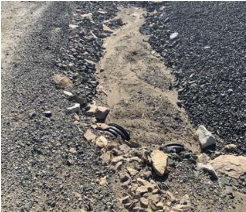
LY-RA-01a: Sediment accumulated in apron. Sediment removal is part of the 2021 inspection maintenance items scheduled.
