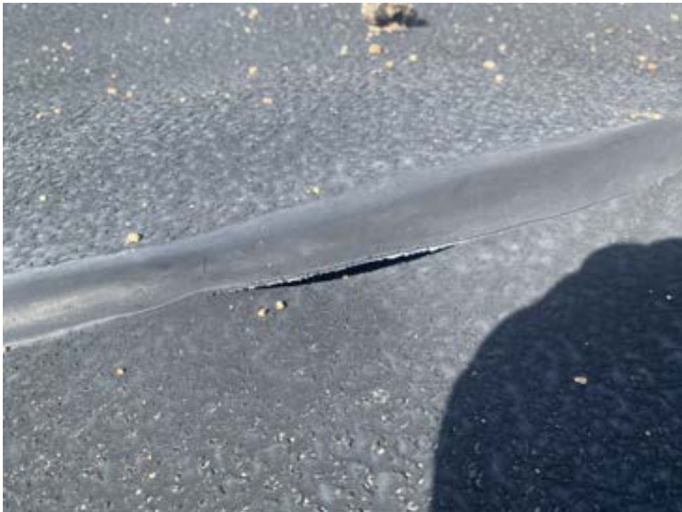
LY-PND-01: New tear in liner (Two liner tears from 2021 inspection still present).
