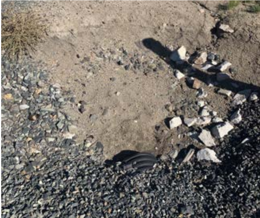
LY-RA-01b: Sediment accumulated in apron. Sediment removal is part of the 2021 inspection maintenance items scheduled.
