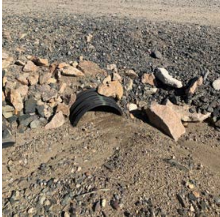
LY-HDPE-03: Sediment accumulation at inlet end of pipe. Sediment removal is part of the 2021 inspection maintenance items scheduled.
