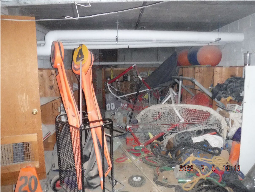
Photograph: 1 View of basement storage area, from bottom of stairwell, facing south.
