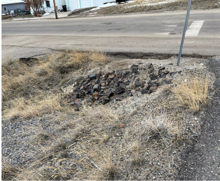
Photograph 4: Erosion and staining on the west side of site next to Montana Street looking west.
