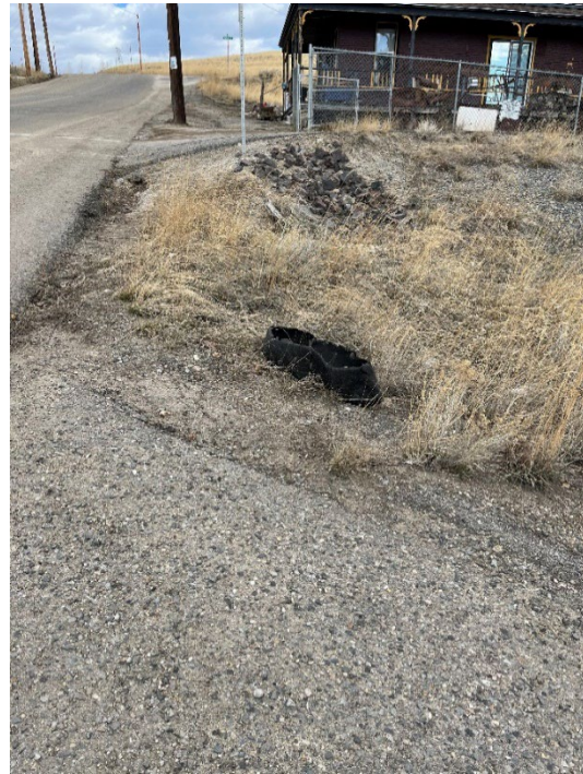
Photograph 6: Erosion next to Montana Street looking north.
