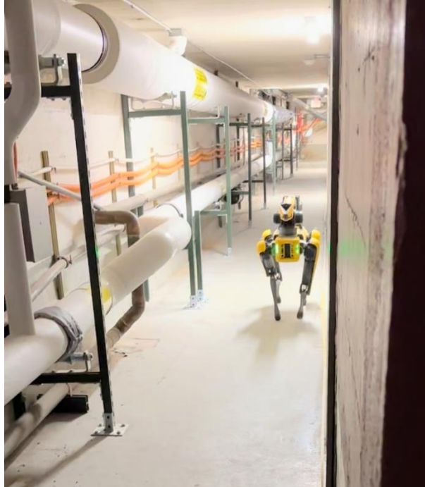
Figure 19: SPOT in Indoor Tunnel
