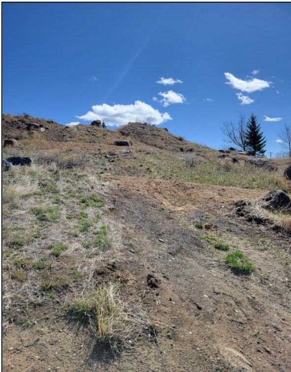
Photograph 5: Temporary Dirt Berms Installed by BSB to Mitigate Sediment Transportation through the Site and onto the Roadway.
