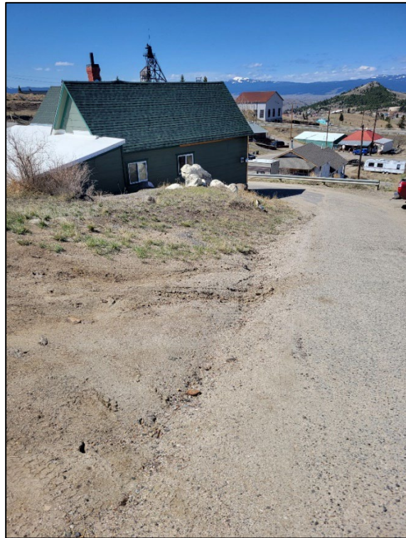
Photograph 6: Storm Water is Eroding onto and under the Roadway.
