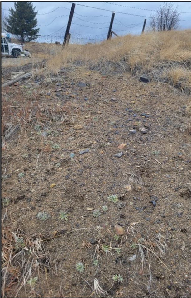
Photograph 1: Barren Areas with Erosion Toward North Main Street.
