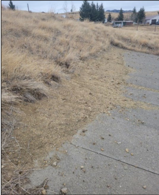
Photograph 3: Erosion onto North Edge of Shaft.
