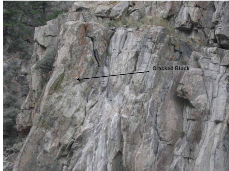
Figure 4: Photo taken of the cracked block by NTL/Terracon employee in 2010 (NTL/Terracon 2011).
