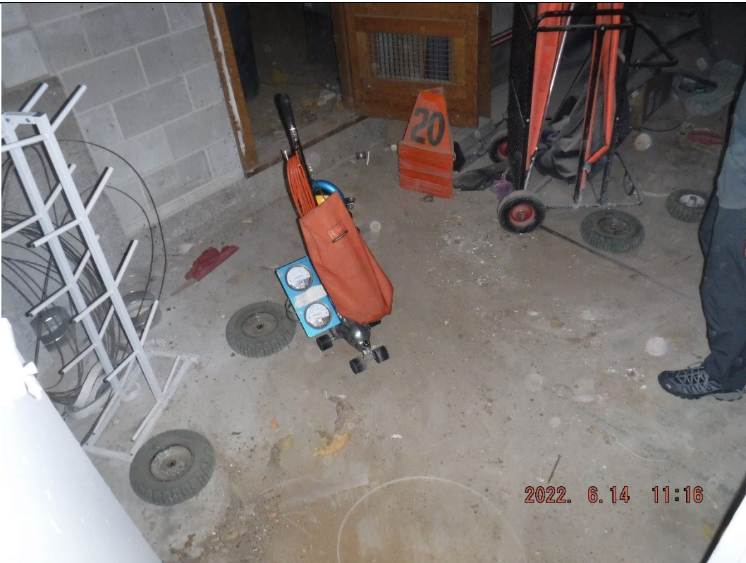
Photograph: 2 View of basement storage area floor, facing towards doorway that leads to eastern crawl space, facing southeast.
