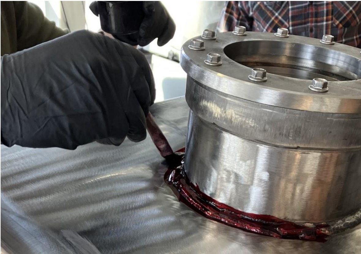
Figure 28: Welding Services Inc. technician applying dye penetrant for weld crack and porosity inspection.
