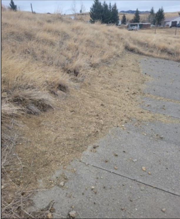
Photograph 3: Erosion onto North Edge of Shaft.
