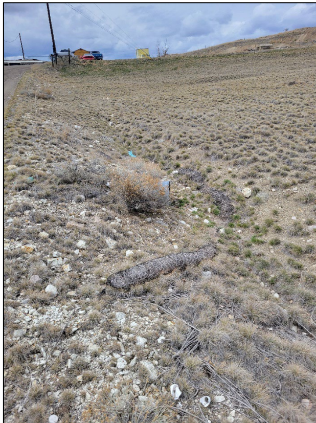
Photograph 5: Off-Site Translocation of Material through Culvert. Previous Sediment control has deteriorated.
