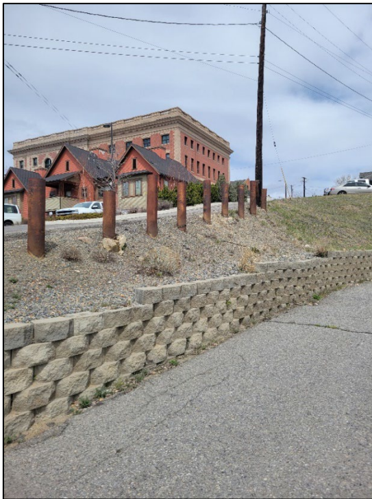
Photograph 2: Butte-Silver Bow Noted a Collapsed Steam Line.
