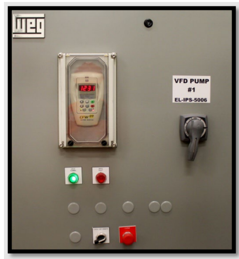
Photograph 9. IPS VFD Panel
