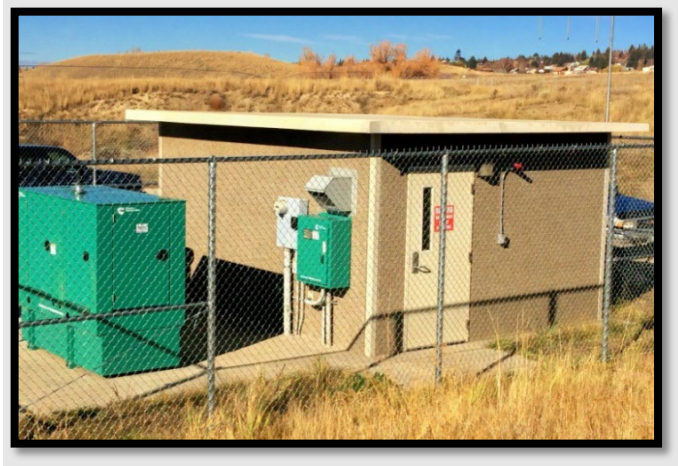
Photograph 4. West Camp Pump Station.
