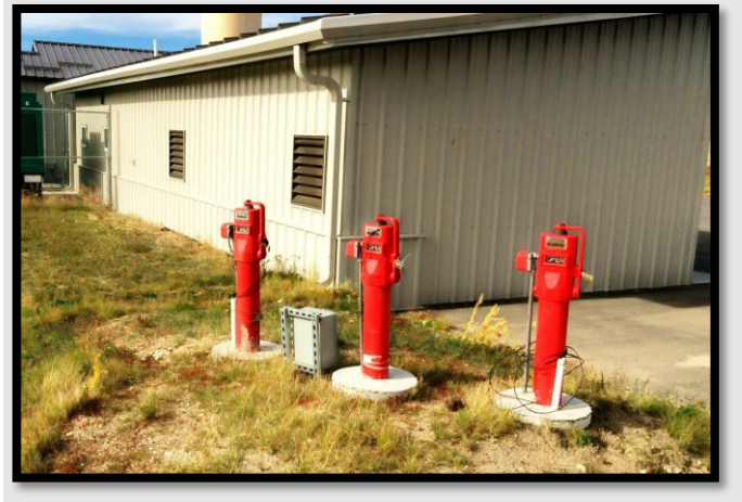
Photograph 7. Influent Valve Indicators
