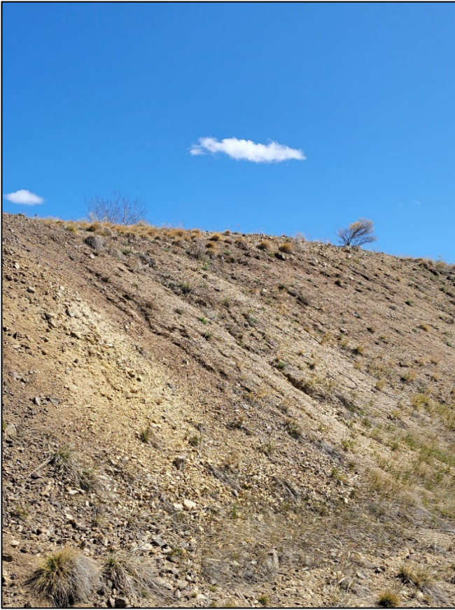
Photograph 3: Erosion and Staining Along South Slope.
