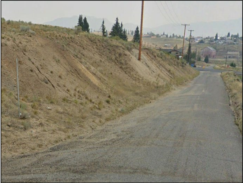
Photograph 2: Steep Slopes with Heavy Erosion onto Road.
