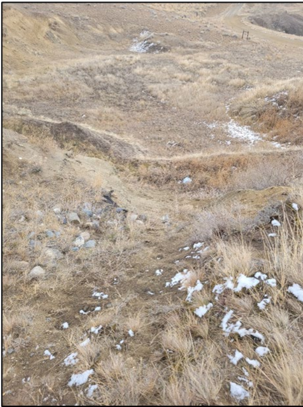
Photograph 3: Gully Developing on North Slope from Possible Storm Water Controls
