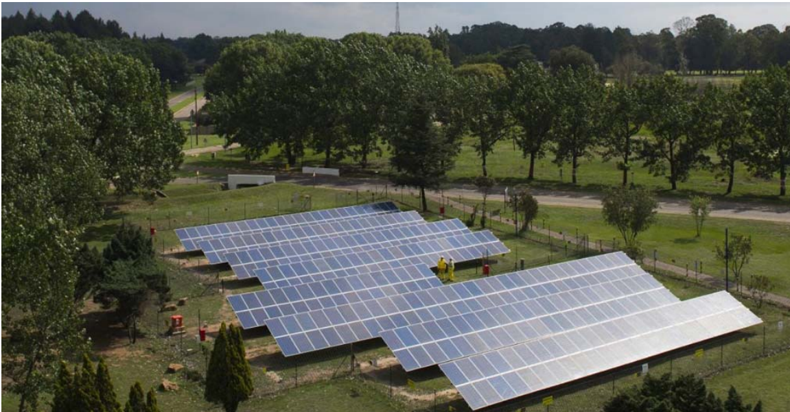
Figure 7: Solar panels installed on a mine site (Anglo American, 2019)
