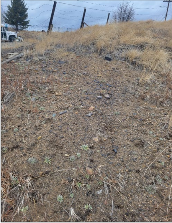
Photograph 1: Barren Areas with Erosion Toward North Main Street.
