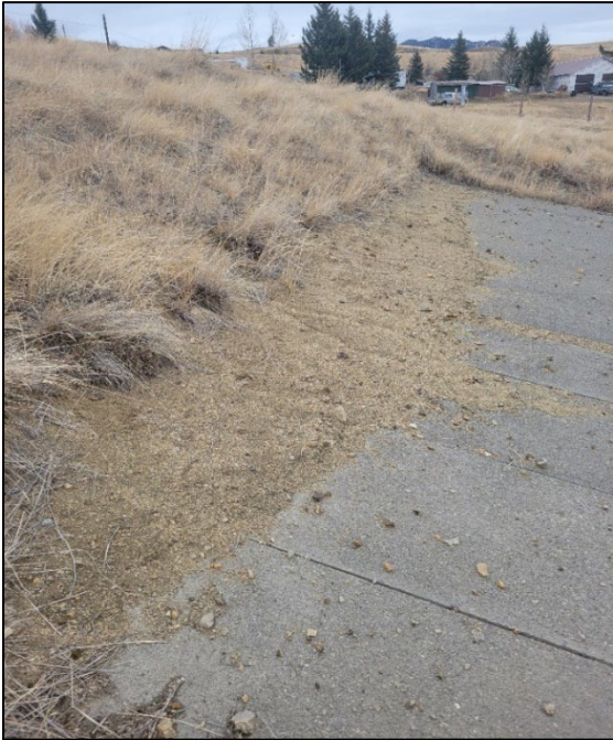
Photograph 3: Erosion onto North Edge of Shaft.
