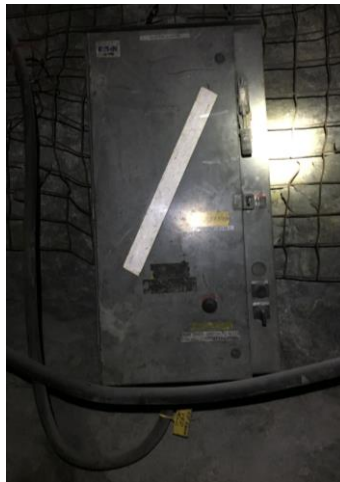
Figure 16. A power station located on the wall along the flight path may have introduced magnetic interference to the UAV's compass.
