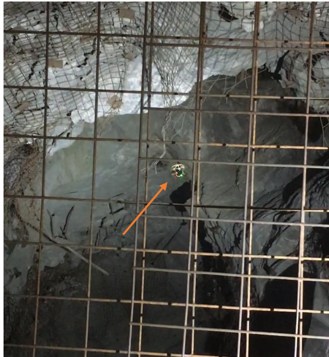
Figure 20: The Elios was piloted from behind a barricade (metal mesh shown in image) toward the ventilation raise, which is located directly above the Elios.
