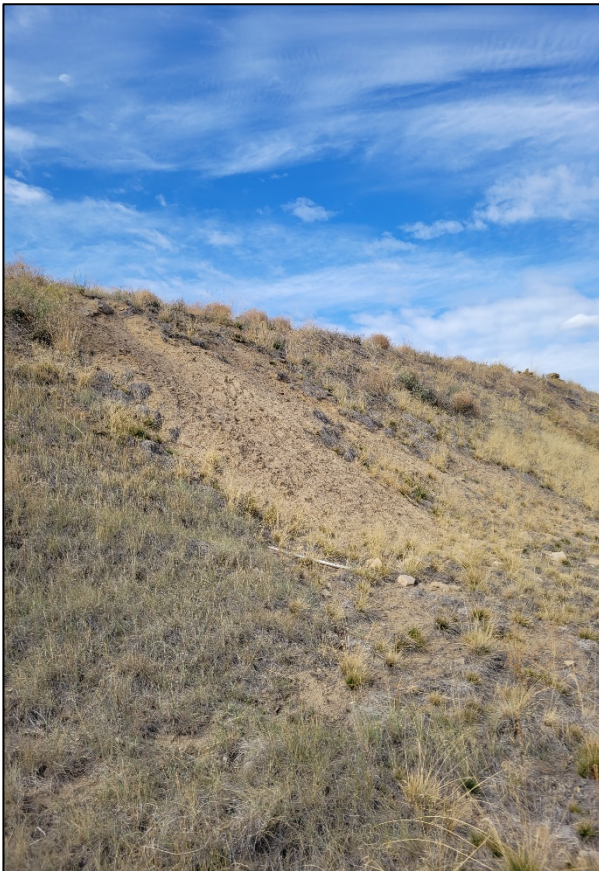
Photograph 1. Possible Mining Waste Erosion
