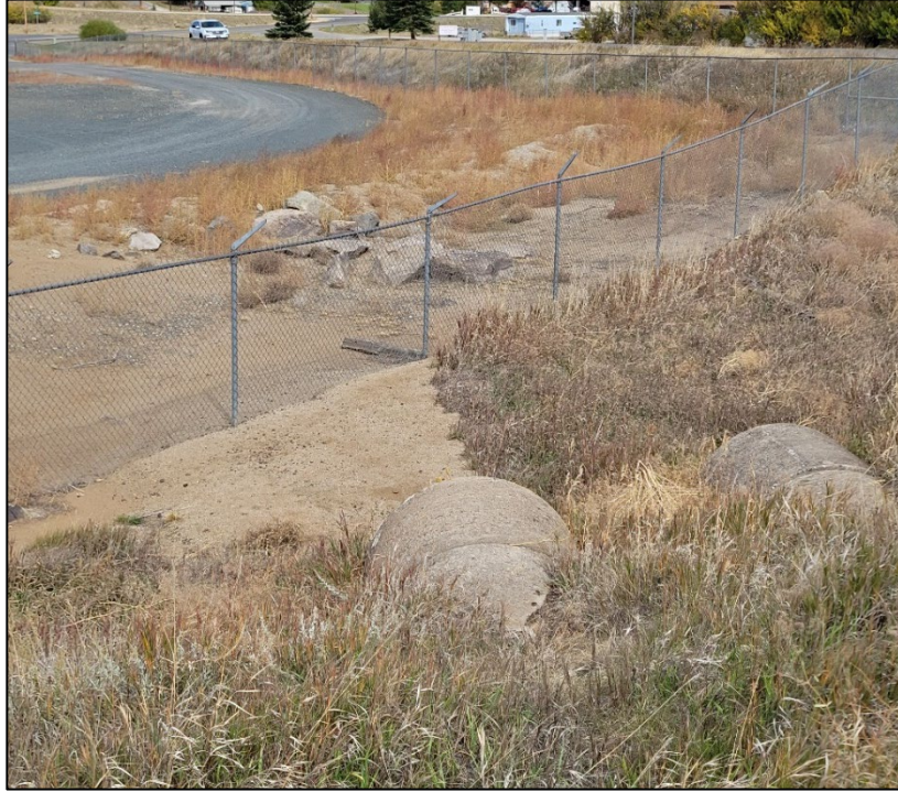
Photograph 9. East Culvert Sediment Deposition from South Storm Water Ditch
