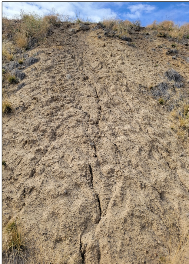
Photograph 2. Erosion Rills on Possible Mining Waste Bare Area
