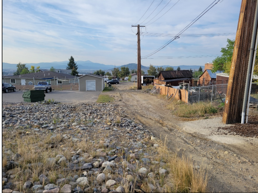
Photograph 2. Storm Water Flows Causing Rills that Transport Material to the South End of the Alleyway.
