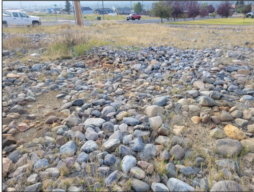
Photograph 1. Possible Mining Waste Leaching through Rock Cap
