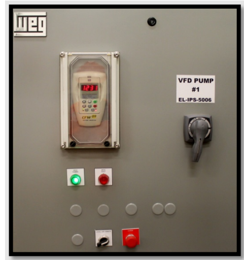
Photograph 9. IPS VFD Panel
