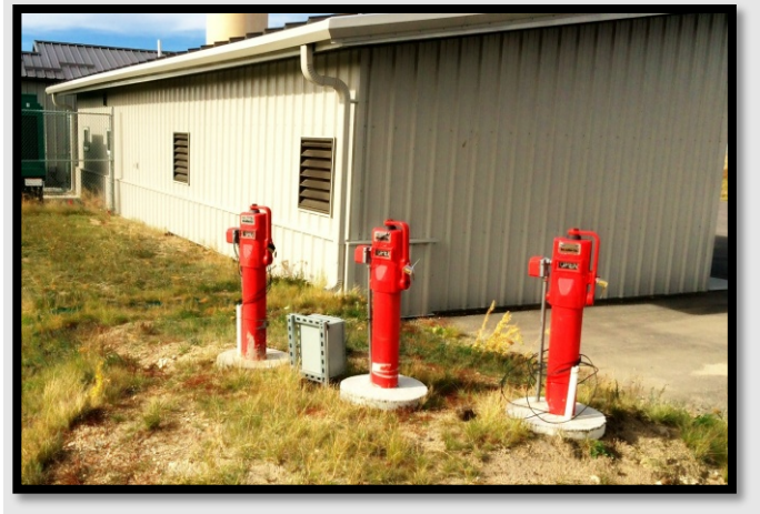
Photograph 7. Influent Valve Indicators
