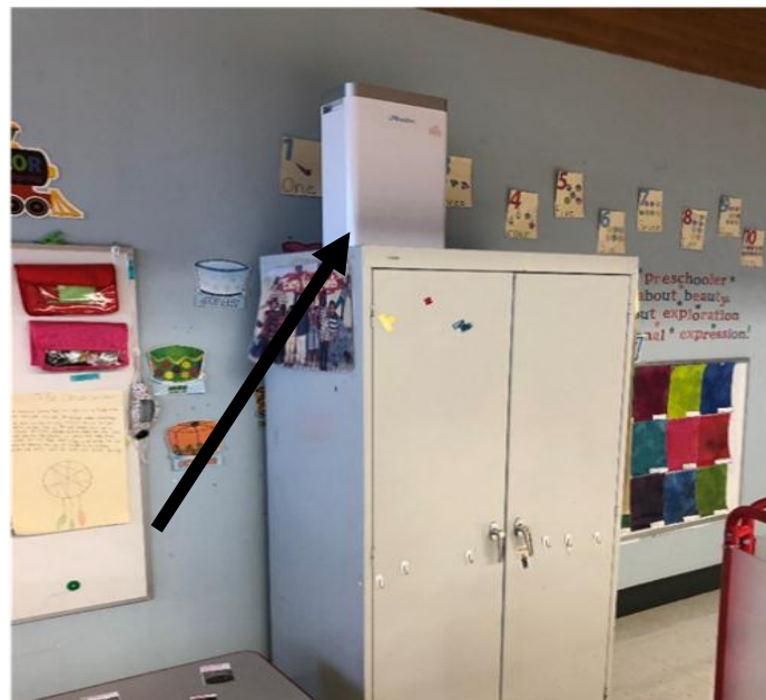
Figure 9. PAC Setup @ Facility 3
