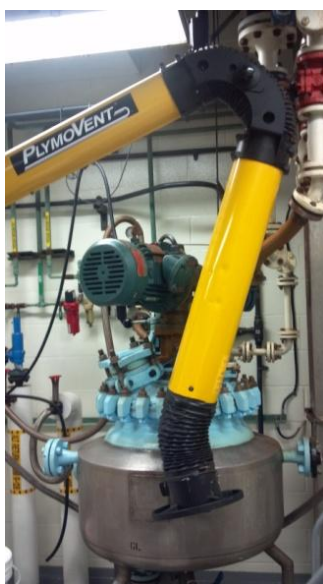
Figure 3: Movable ventilation duct.
