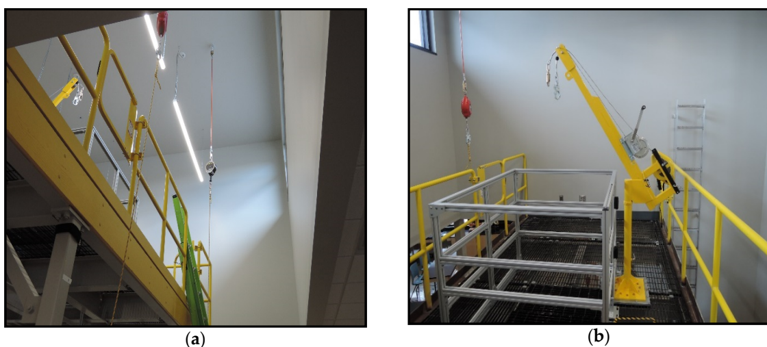
Figure 2. Personal fall arrest anchorages: (a) ceiling mounted anchor, (b) davit on the mezzanine.
