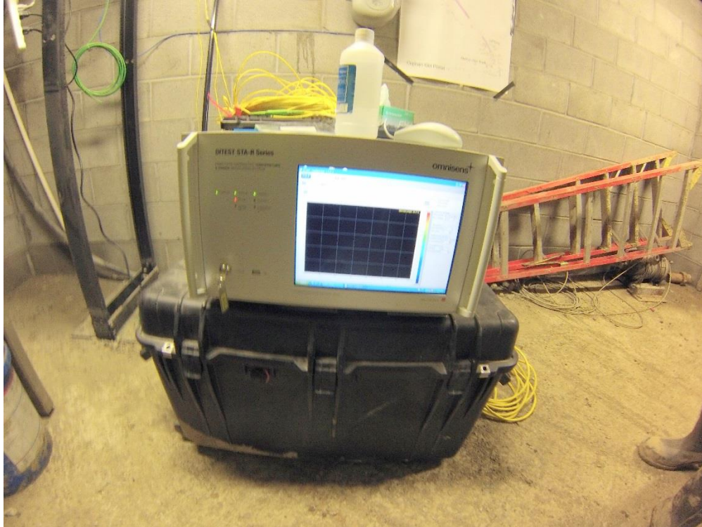
Figure 4. Pictured above is an Omnisens DITEST STA-R™ high-performance Brillouin-based fiber optic distributed temperature and strain analyzer collecting temperature data in the Orphan Boy mine shaft.
