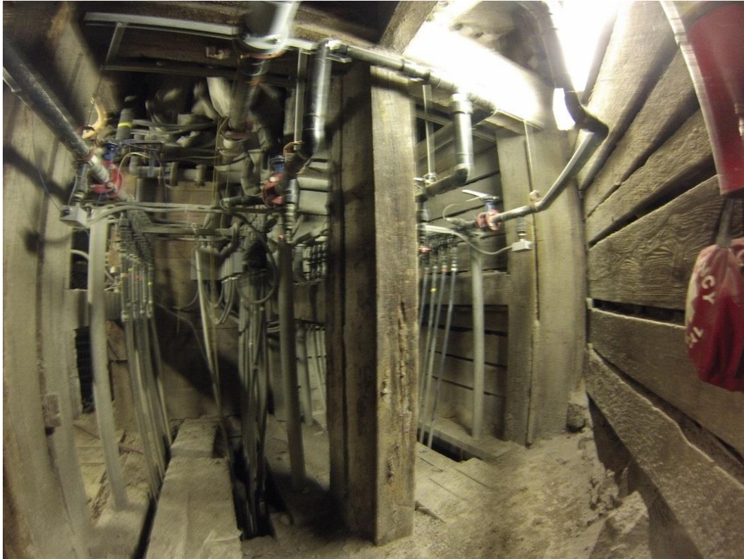
Figure 2. Pictured is the closed-loop heat pump as it sits above the Orphan Boy mine shaft in Butte, Montana, USA. The 2011 installation of this mine-based heat pump was funded by the American Recovery and Reinvestment Act of 2009.
